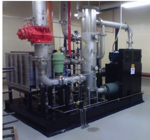
Figure 3-4 Representative Biogas Booster System
