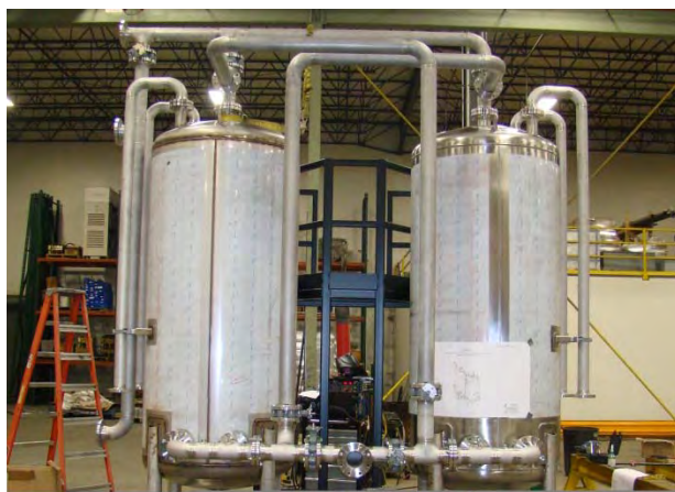
Figure 5-4 Representative Siloxane Treatment Vessels
